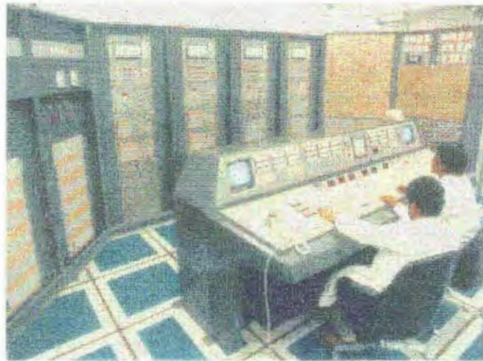
Figura 11: Sala de Control del Reactor Nuclear RP-10.
